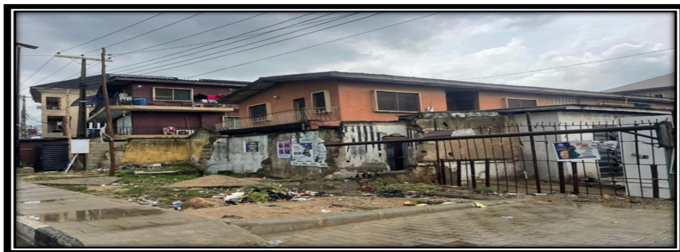
Plate 1: A Partial demolished of building at Kemist area that that was poorly handled
